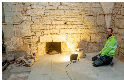
Fig. 4. Workman Heigo Leemet at the opening to the chamber found in the Sturvolt wall after the removal of the plaster covering the wall. The well's door opening remained partially concealed by the cellar's current floor.
