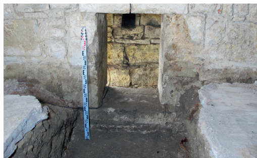
Fig. 5. The cellar's original floor was around 75 cm lower than the current floor (1985). A wooden hatch covered the well's door opening ( 100 \times 70 cm). The locations of its hinges are still identifiable. A small illumination opening can be seen in the well's outer wall in the background.
